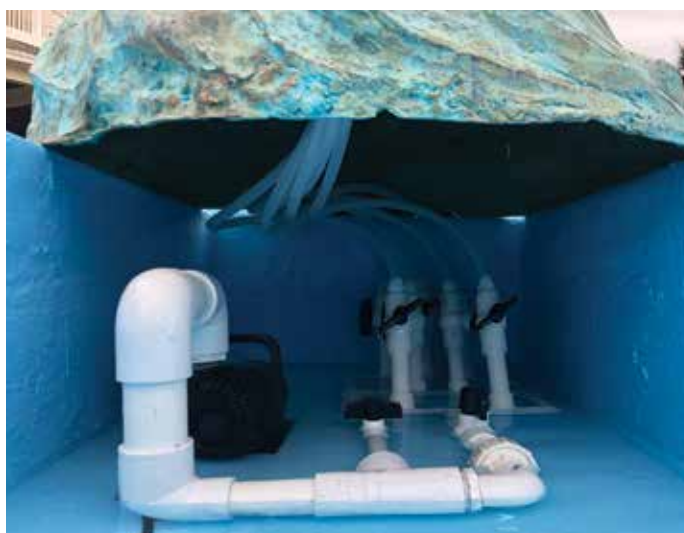
PVC new piping and distribution manifold
